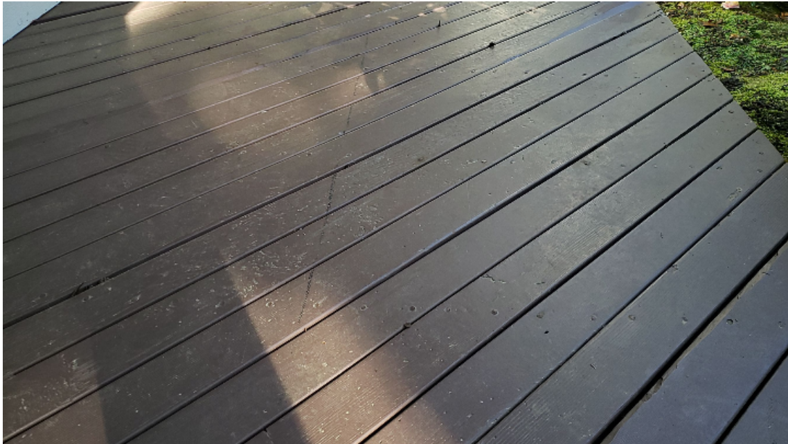
Building Exterior - Deck, Surface, 25% Replace
